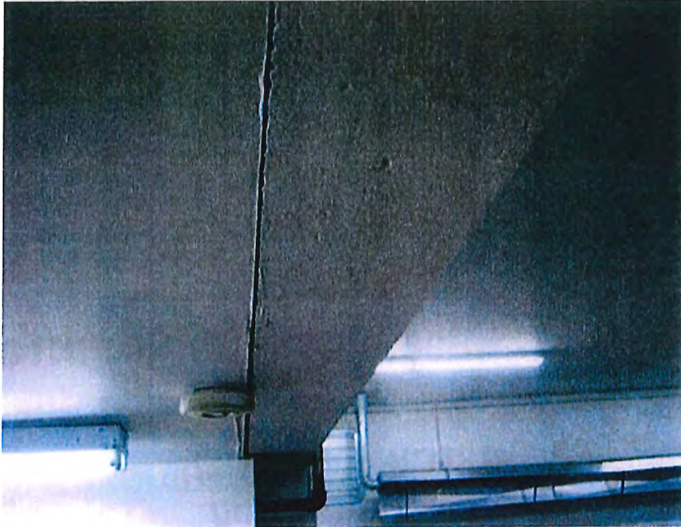
Figure F.7 Bottom of existing header at truck bay location showing concrete (shown as a wood beam on existing drawings)
