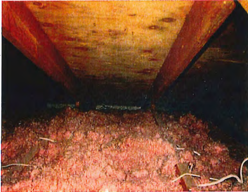
Figure F.3 Existing roof trusses at end support to sill plate on top of masonry wall (not adequate shear transfer from plywood sheathing to sill plate).
