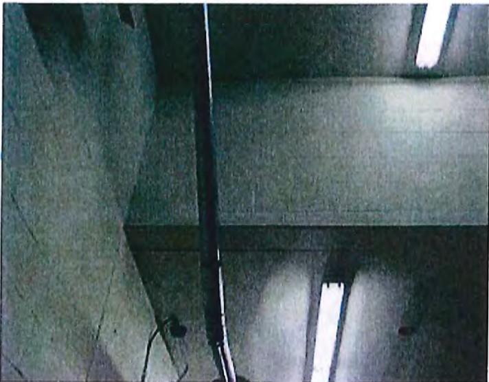
Figure F.6 Existing header at truck bay location built as concrete (shown as a wood beam on drawings)
