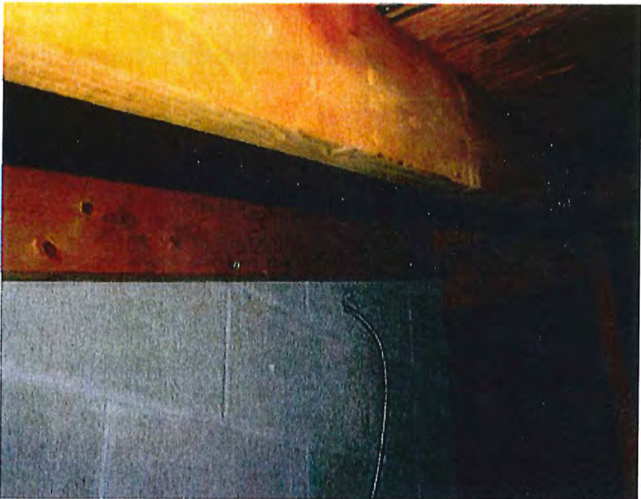
Figure F.1 Existing wood roof ledger connection to masonry walls (not properly connected for shear transfer)
