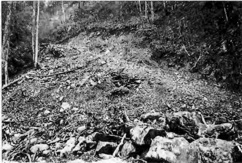
Photo 1. View looking northeast from Rockwell Drive and Lillooet Avenue. Start of steep (55°) road slope.
