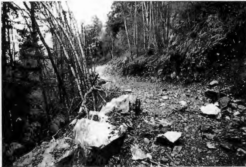
Photo 2. Looking north from point HL10 at the constructed road. Cutslopes on the east is unstable, large blocks on the west of the rock (side-casted) poses a hazard.
