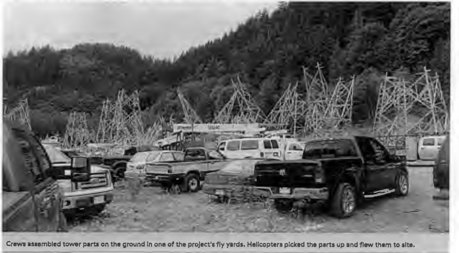
Crews assembled tower parts on the ground in one of the project's fly yards. Helicopters picked the parts up and flew them to site.
