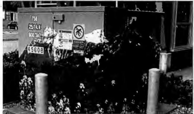
Decorative wraps on pad-mounted equipment in Chilliwack.
