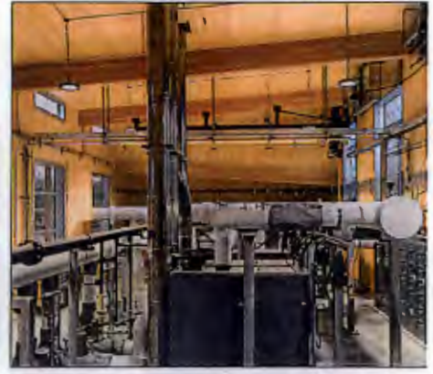
LMLGA -- Lower Mainland Local Government Association: City of Richmond for the Alexandra District Energy Building
