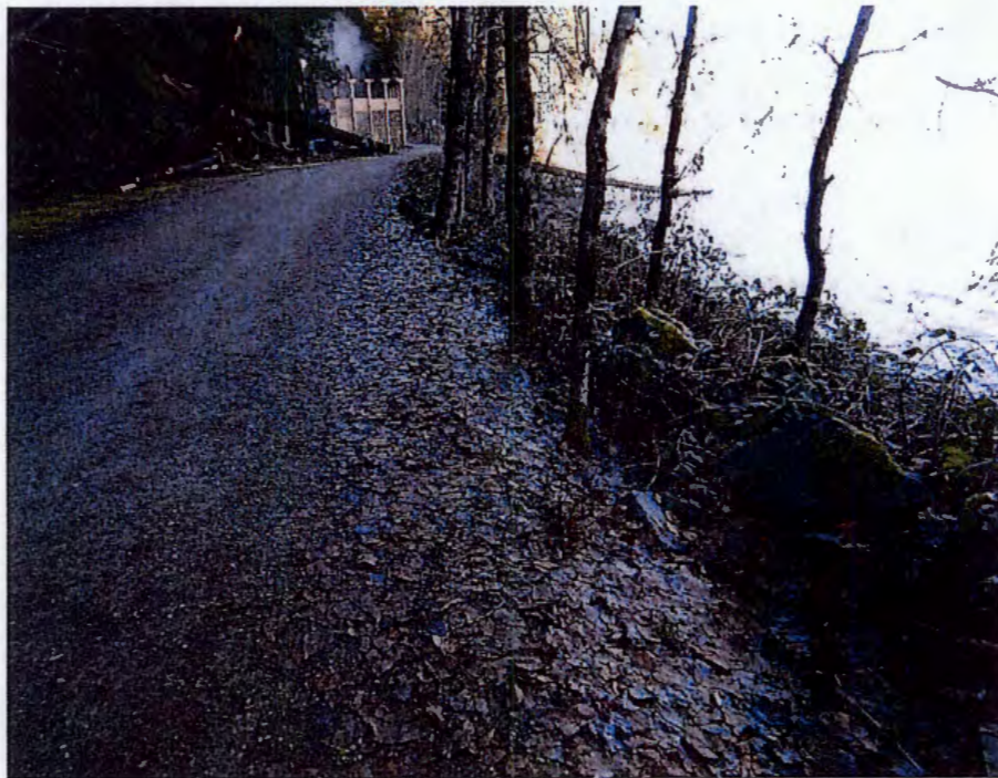
Figure 3.4 Zone 2. Access road to the WWTP includes tree growing at the top of the armoured slope.
