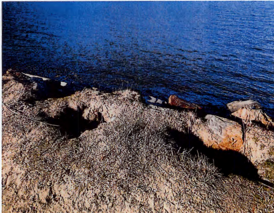
Figure 3.16 Zone 5 – Observed erosion at the top of the riprap slope on the lagoon berm.
