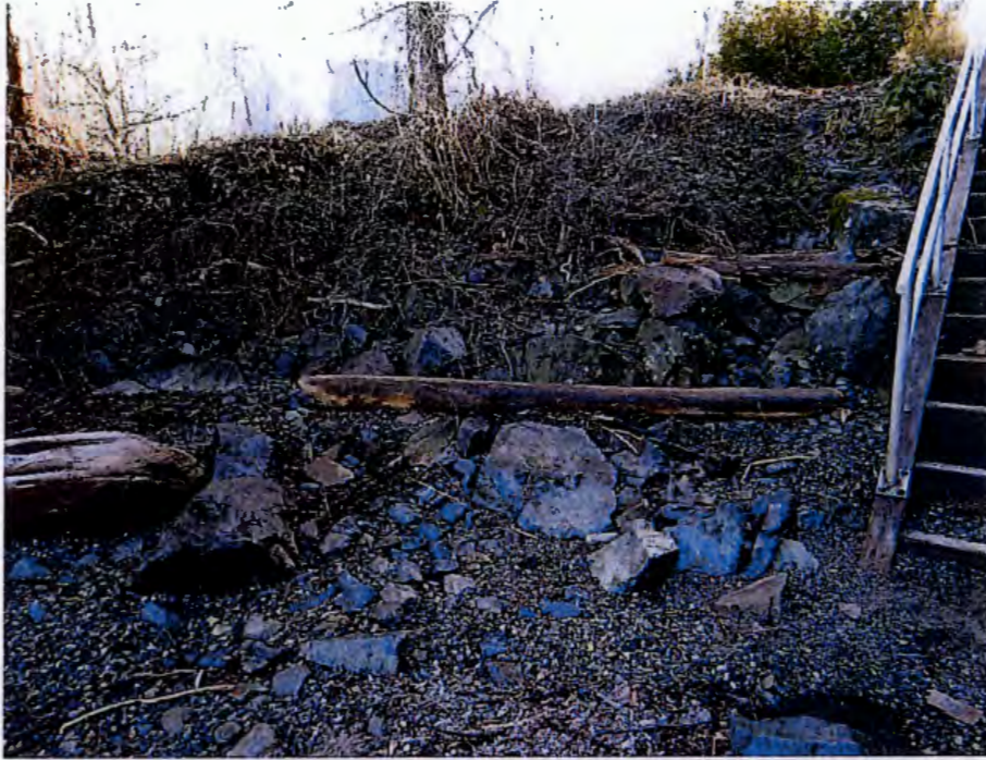
Figure 3.8 Zone 3 – Invasive species covering the deteriorated riprap slope.
