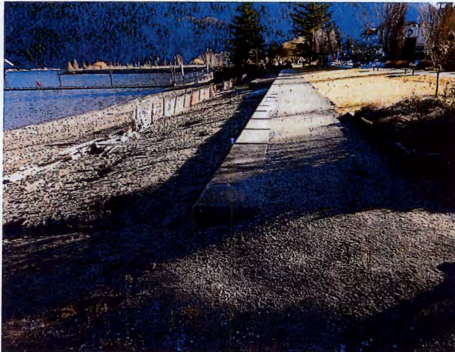
Figure 3.9 Zone 4 – Beach with lock-blocks (scour in front of lock-block is visible) and wooden slat fencing.
