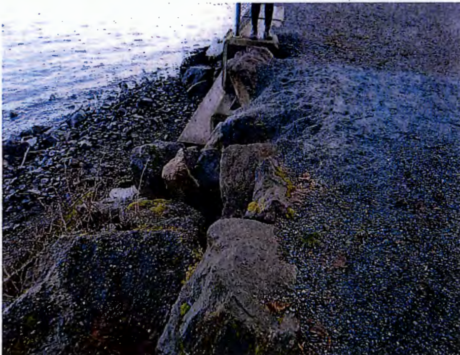
Figure 3.6 Zone 2 – Repairs to the top of the slope adjacent to the Miami Creek outlet.
