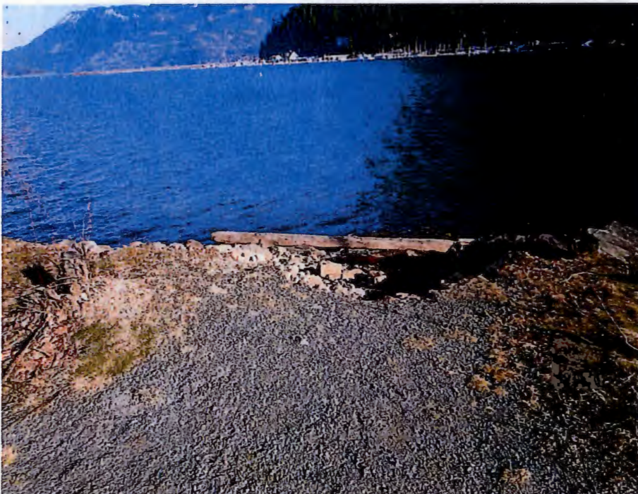
Figure 3.18 Zone 5 – Observed location of erosion in the lagoon berm.
