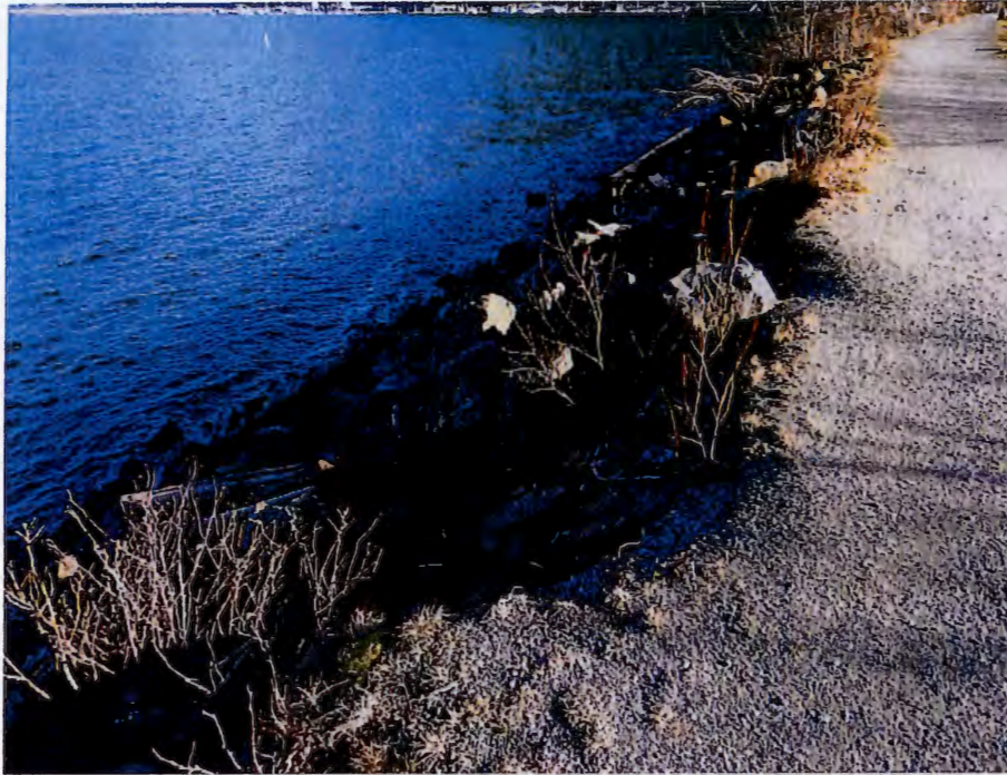
Figure 3.17 Zone 5 – Variation in sizes of riprap on the offshore slope of the lagoon berm.
