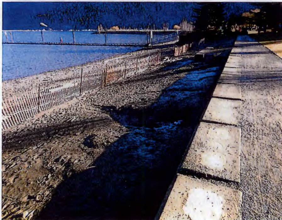
Figure 3.13 Zone 4 – Lock-block wall with scour occurring in front.
