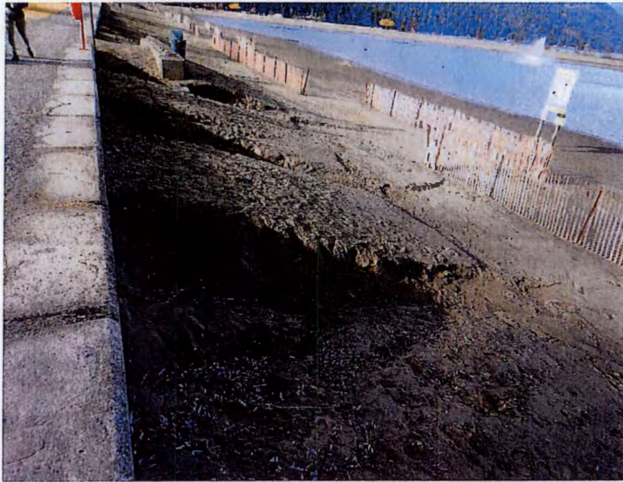
Figure 3.19 Zone 5 - Existing lock-block wall and wooden slat fencing along the dike in front of the lagoon with severe erosion.
