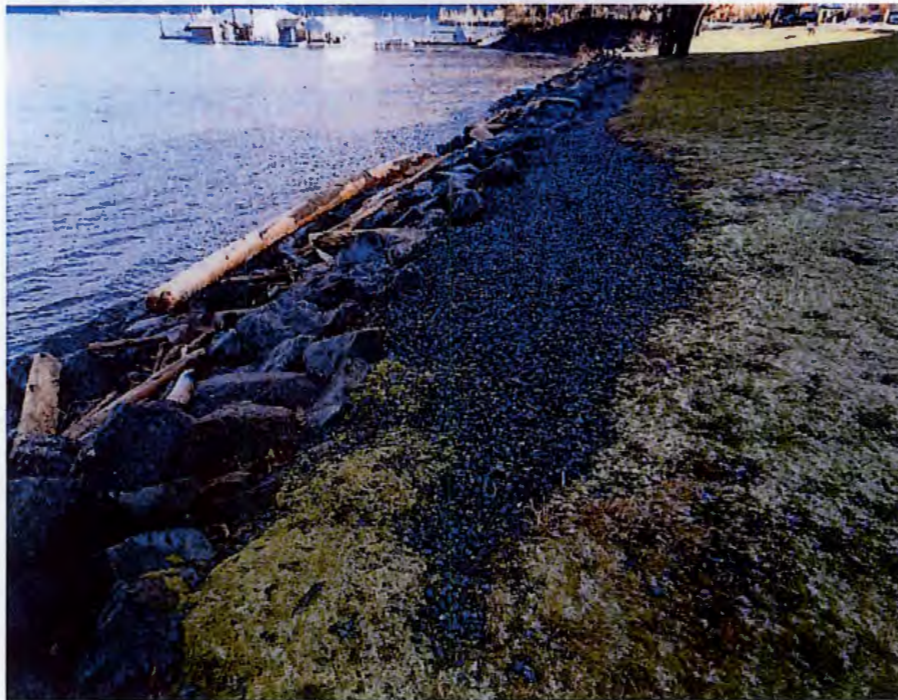
Figure 3.11 Zone 3 – Assumed repairs to top of riprap in front of Harrison Hot Springs.
