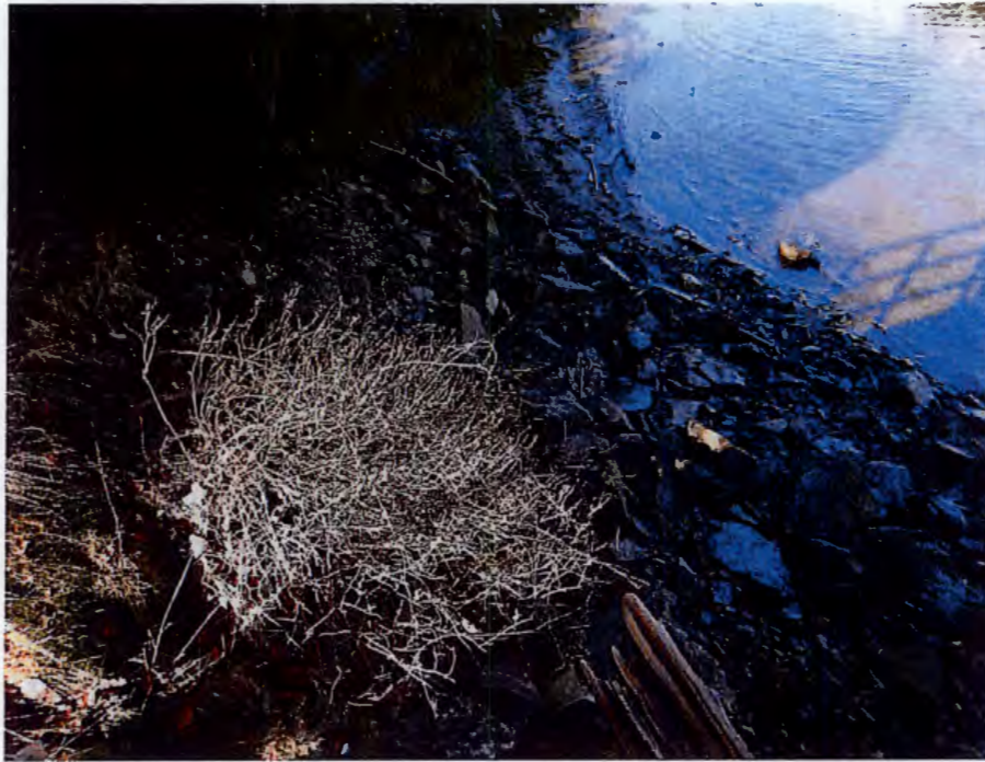
Figure 3.10 Zone 3 – Riprap in poor condition at the eastern extent of zone 3 adjacent to the marina access peninsula.
