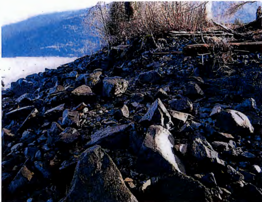
Figure 3.9 Zone 3 – Deteriorated riprap slope
