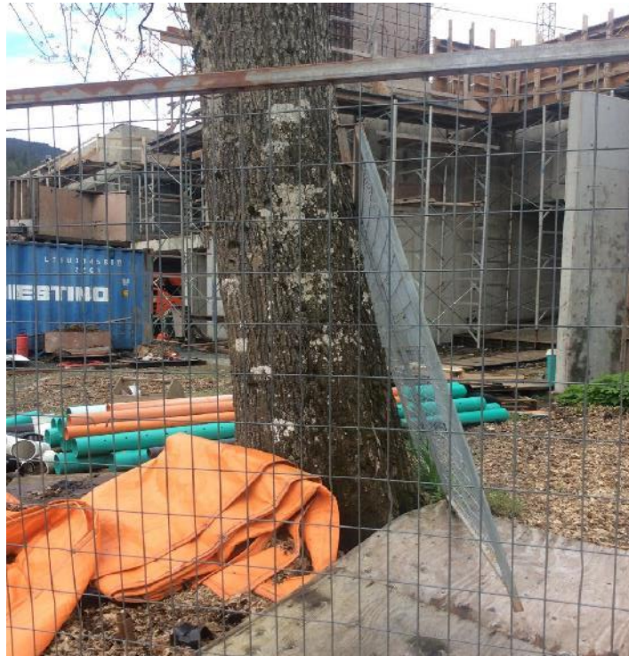
Figure 5. Construction piled against one of the large oaks on Lillooet Road; no tree protection present.
