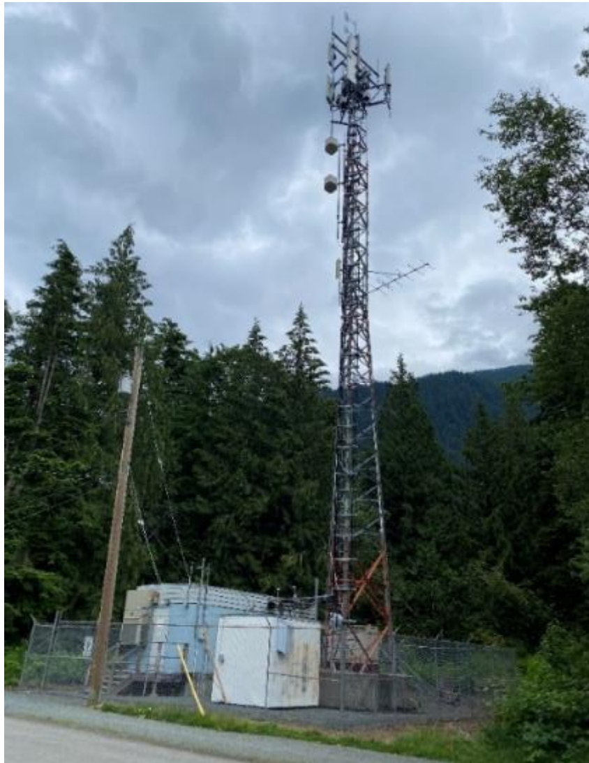
Figure 20. The communications tower located in the East Sector Lands could be impacted by a nearby tree failure.
