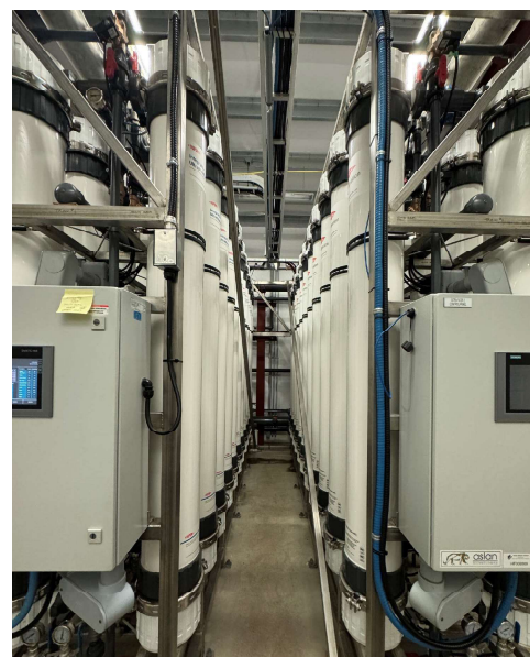
Figure 14: Ultrafiltration Membranes, Two Trains
