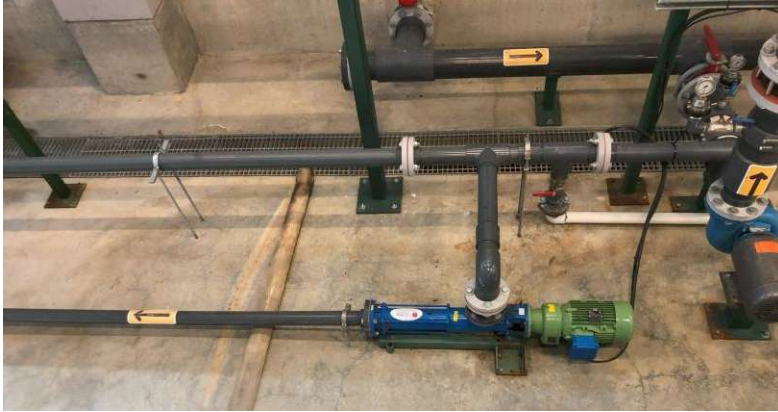
Figure 15. WAS transfer pump to the Centrifuge
