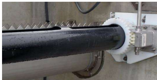
Figure 25. Rotating Scum Removal System
