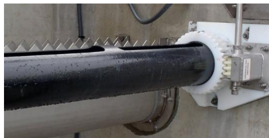
Figure 25. Rotating Scum Removal System
