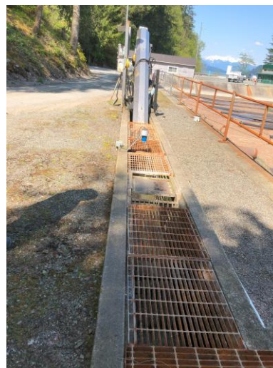
Figure 9. Influent Channel with Helisieve. Corroded grating and bioreactor railing.
