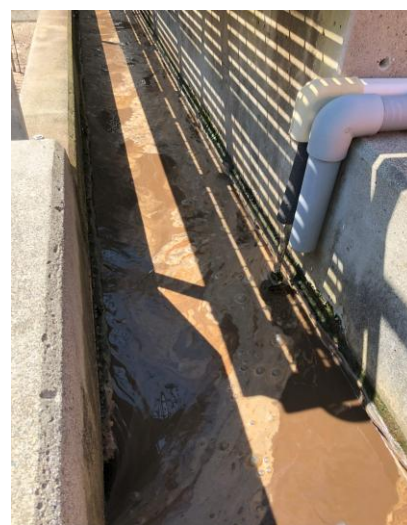
Figure 13. Mixed Liquor Effluent Channel. Promotes recirculation of floating sludge.
