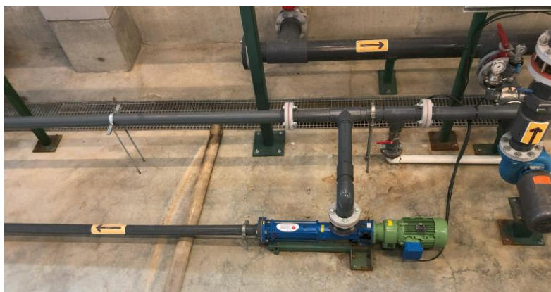
Figure 15. WAS transfer pump to the Centrifuge
